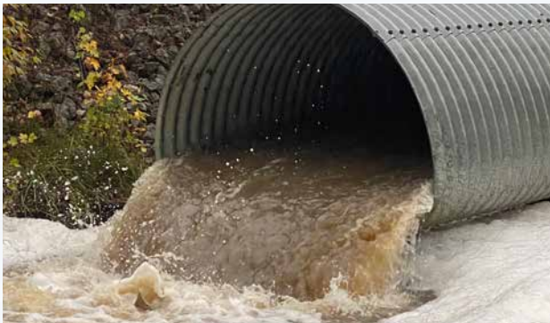
Dillon Creek inflow into Enchanted Hills after a large October 2021 rain.
